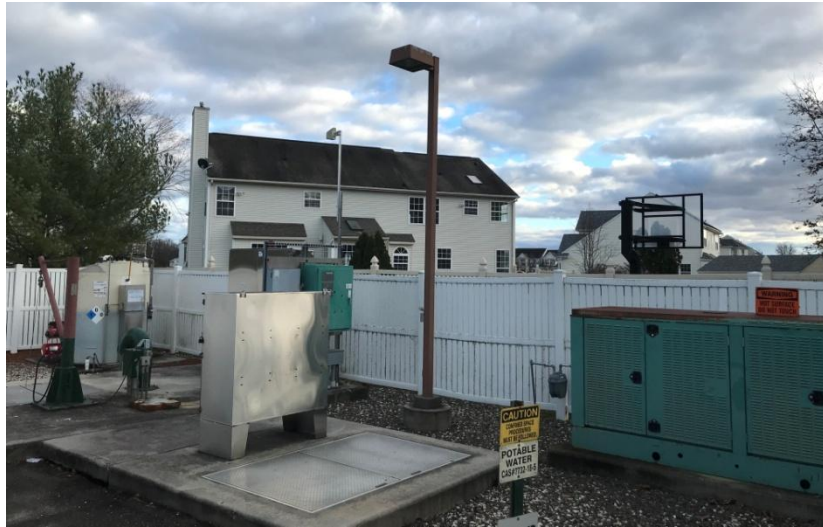
Figure 12: View looking toward the Arbours Pump Station from the southeasterly corner of the pump station lot.
