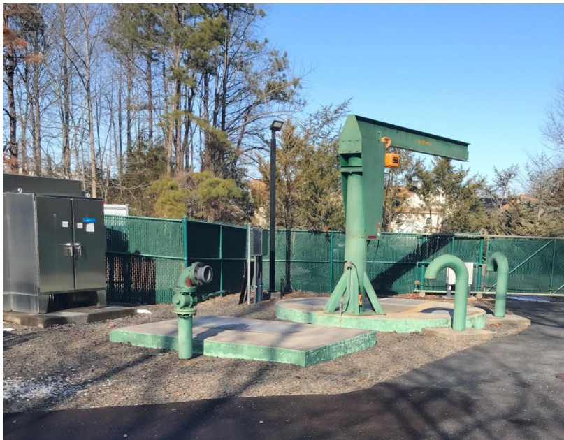
Figure 11: View looking toward the Lake Avenue Pump Station from the rear of the site. Note the jib crane positioned over the wet well.
