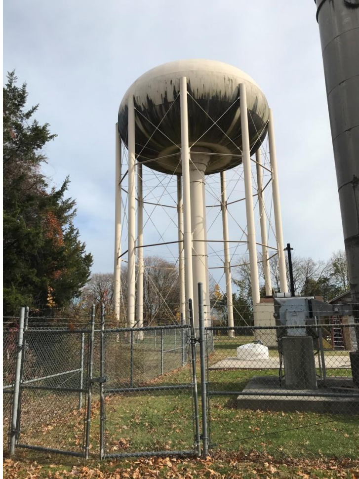
Figure 3: View looking in a northeasterly direction toward the Corkery Lane Water Storage Tank showing dark mold on the bottom of the bowl.
