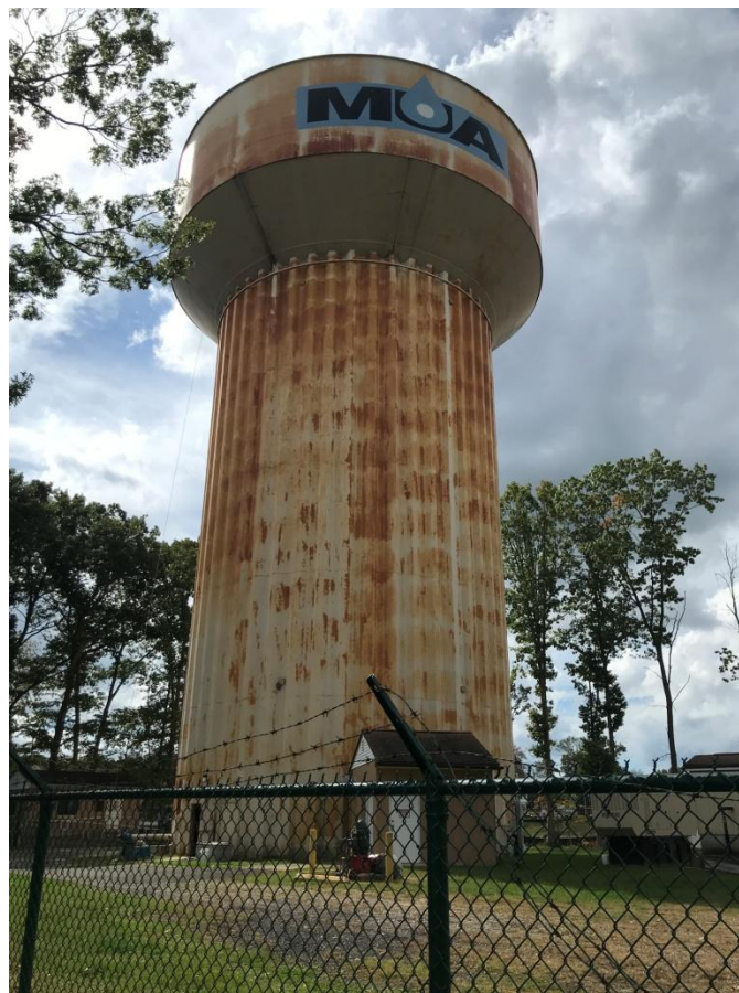
Figure 1: View looking in a southerly direction toward the Knights of Columbus Water Storage Tank from MMUA property. Note corrosion of the column and storage bowl.
