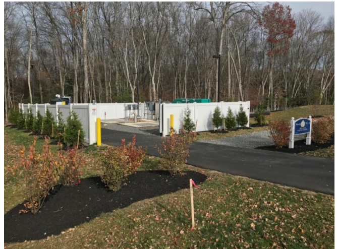
Figure 10b: View looking toward new Mink Lane Pump Station from Acorn Lane.
