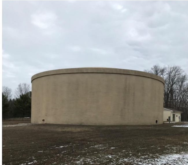
Figure 5: View looking in a northerly direction toward the South Black Horse Pike Water Storage Facility.
