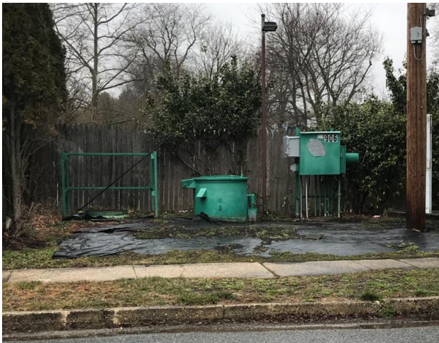
Figure 10a: View looking toward the Chelsea Farms Pump Station from the Frederick Street.
