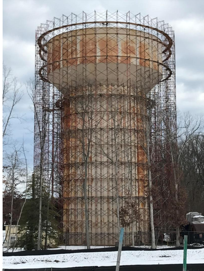
Figure 2: View looking in an easterly direction toward the Knights of Columbus Water Storage Tank the adjacent “Grandview Mews” development presently under construction. Scaffolding has been erected to facilitate paint removal and repainting.
